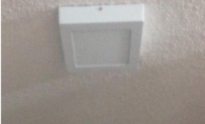
Figura 71. Panel LED atenuable instalado
