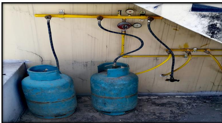
Figura 4. Central de Gas
